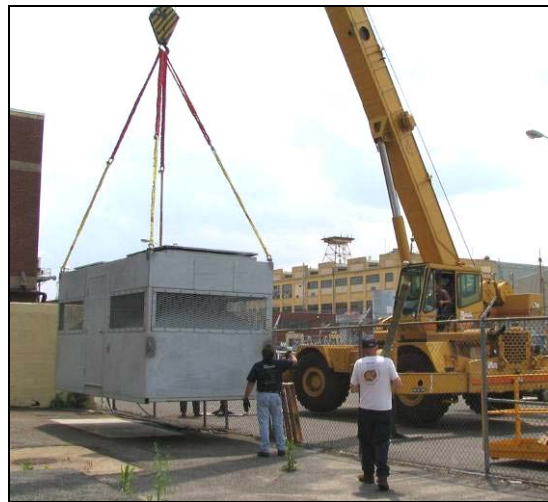
Figure 9. Positioning 3.5 MW resistor load bank for higher power Static Load tests
