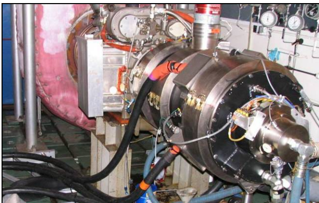
Figure 7. View of high-speed generator installed in turbine test cell with ETF40B engine
